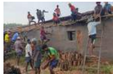
Youth members involved in building houses as part of the livelihood activity
